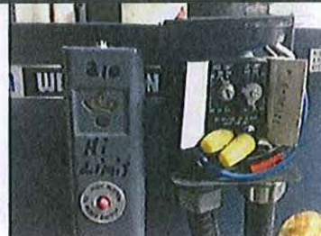
High temperature controller and operating controller for the oil fired boiler M15.1
