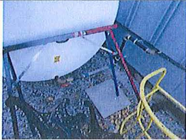
Storage in and around fuel oil tank N8.1
