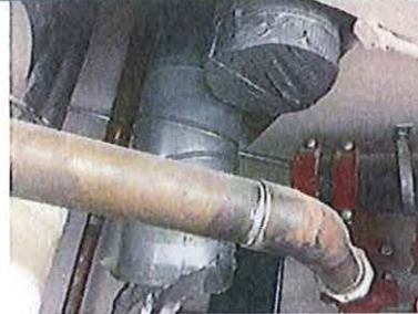
Capped ductwork from the second floor ventilation grilles M10.2
