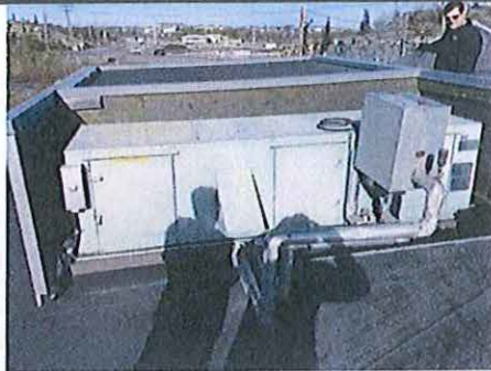
Rooftop Air Handling Unit M9.1
