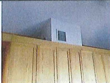
Ventilation grilles in the second floor board room M10.1
