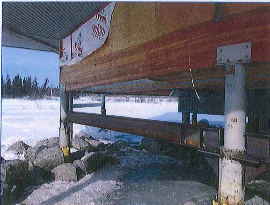
Figure 1: Failed Glulam Beam supporting ramp, installation of substitute wide flange steel beam at lower elevation. This scheme permitted us to remove sections of the original steel pipe pile. Having removed approximately 7" of the intermediate pile, the gap between the broken glulam beam and the steel beam was filled in with a load bearing wall assembly. The surface was sheeted with plywood and covered with galvanized cladding consistent with the original design.
