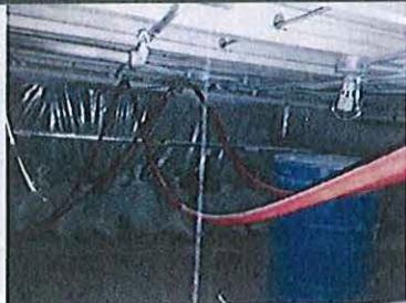
Painted sprinkler head M11.1
