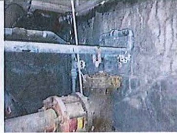
Water service entrance M13.1
