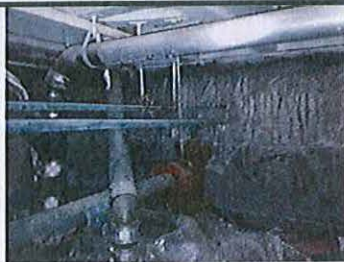
Water service entrance M13.2
