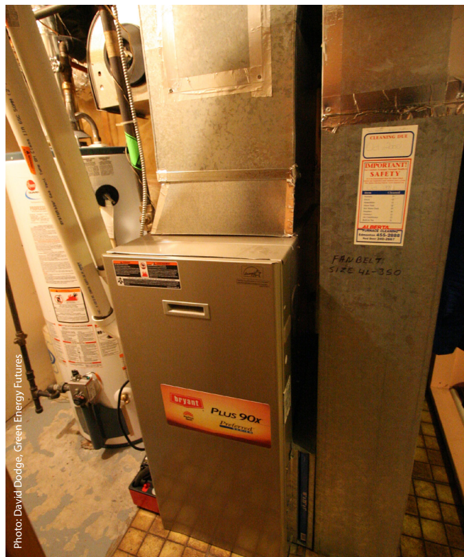
Efficient natural gas furnace
