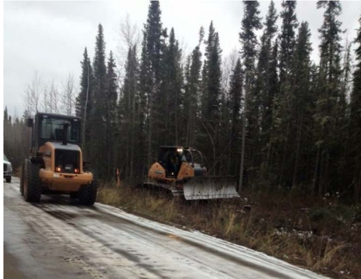
Construction takes place on the Mission Island Access Road in Fort McPherson.
