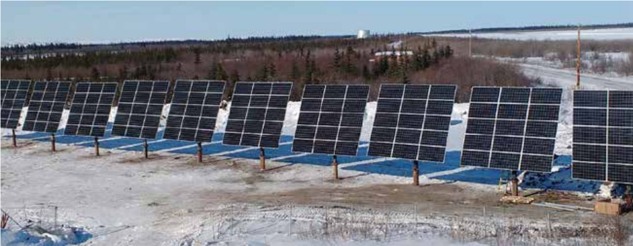
55 kW Solar PV Installation in Aklavik.
