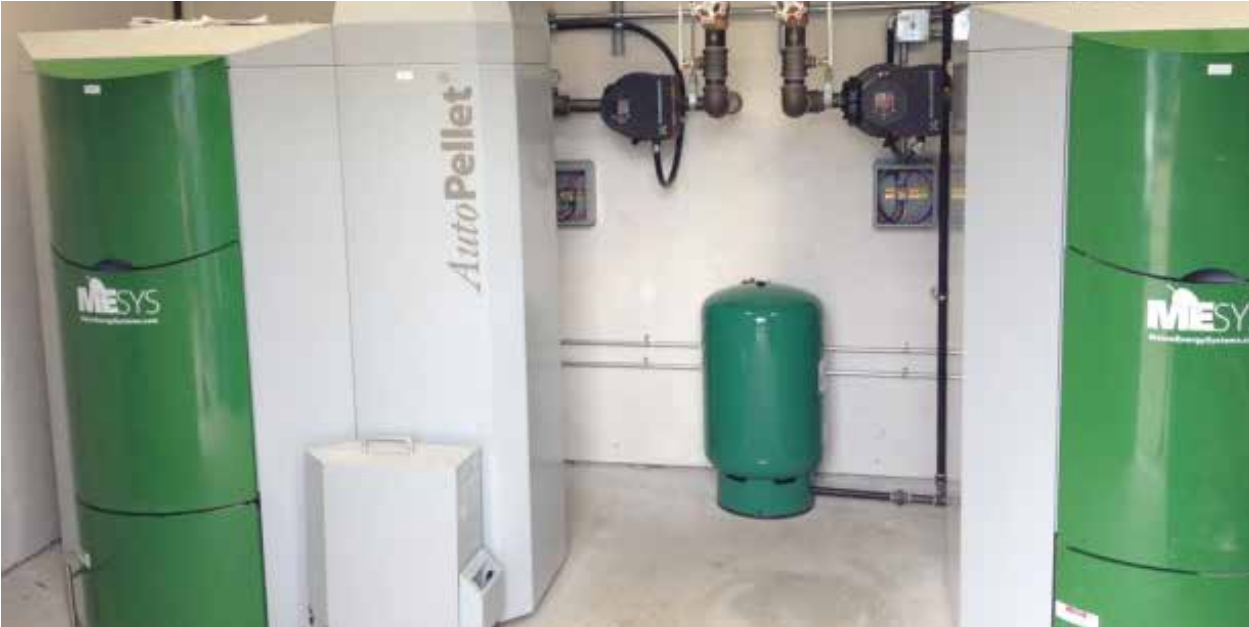
New Pellet Heating System for Fort Simpson's P.R. Contracting Ltd.
