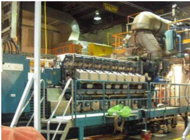
2.5 MW Natural Gas Generator + Exhaust Gas Heat Recovery Unit.
