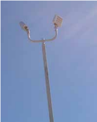
New LED Light Pole.
