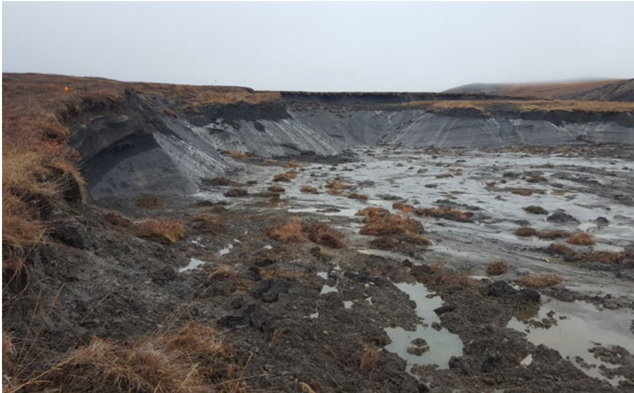
A thaw slump adjacent to the Dempster Highway where permafrost ground temperature monitoring stations have been installed
