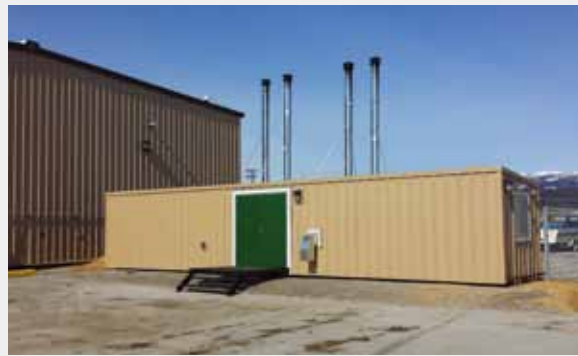
224 kilowatt wood pellet boiler system at the Norman Wells Airport Maintenance Building
