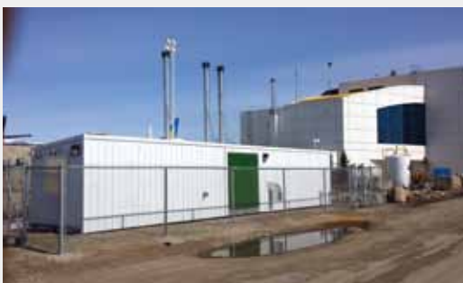
168 kilowatt wood pellet boiler system at the Norman Wells Air Terminal Building
