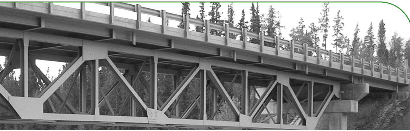
Canada and the GNWT invested $34.5 million in constructing and rehabilitating bridges and culverts since 2002. Additional investments of $64 million are proposed to upgrade, repair, bridges on the NWT highway system.
