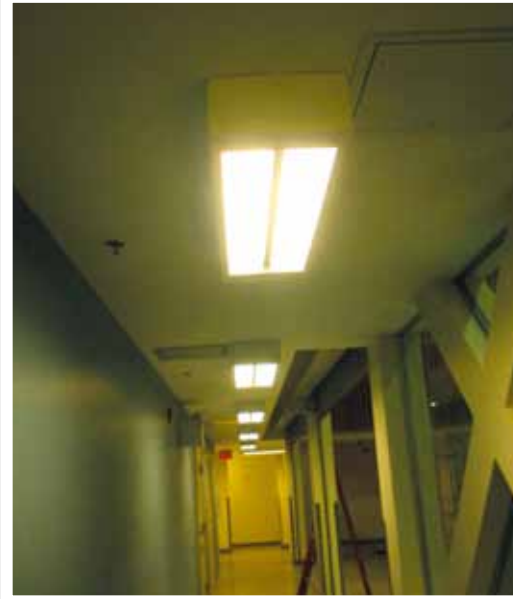
1 x 4 LED fixtures used around perimeter on 1st and 2nd floor with dimmable control for user adjustment to daylight levels.
