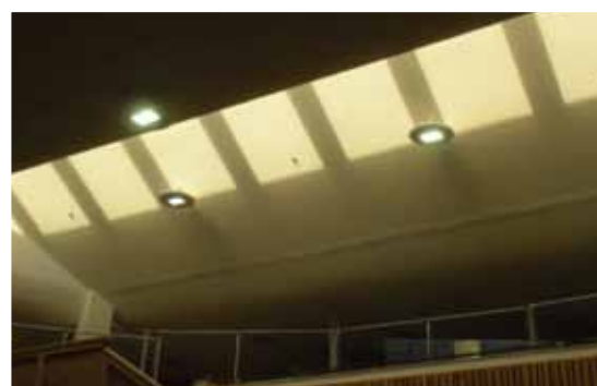
High bay LED fixtures utilized in the Diamond Jenness Secondary School atrium provide sufficient lighting with longer lamp life.
