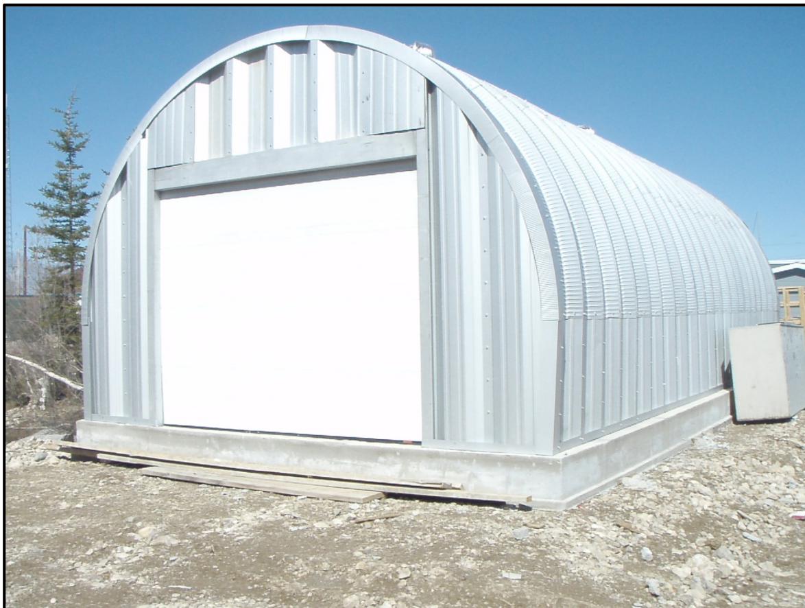
The new depot in Behchoko under construction in 2008, the large rear doors allow for easy removal of fibre “mega” bags containing collected containers.
