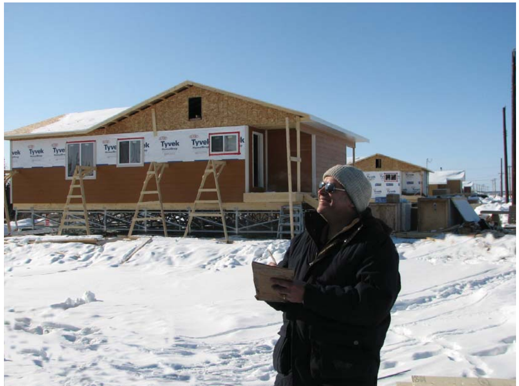
Sahtu District Office Technical Manager, John Kivi , could not be happier to be inspecting new home construction in Fort Good Hope on such a beautiful day.
