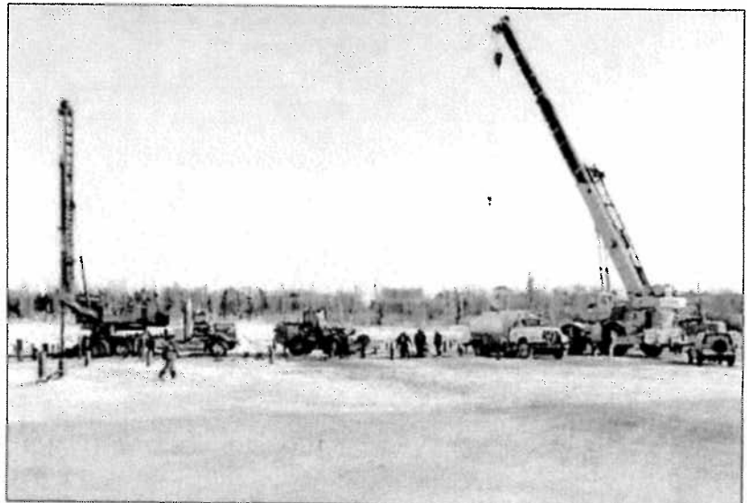
The pilings installation for the Inuvik super school, by Dowland Contracting, began in November and finished in March.
