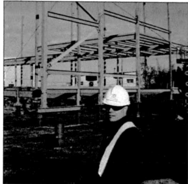
Todd Ingram, senior project officer, oversees the Inuvik school replacement project for the GNWT's Department of Public Works and Services. Here, he stands at the construction site at the start of the installation process for the school's steel superstructure.
