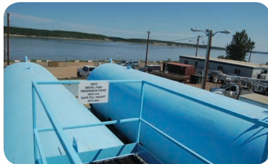
Diesel fuel storage tanks, Fort Simpson.
