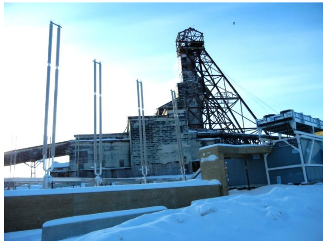
Thermosyphons at Giant Mine
