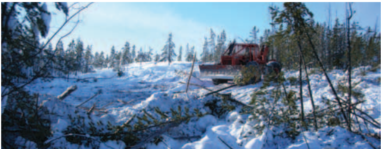
FIGURE 25. Use of a shear blade with a skidder is an acceptable method of clearing in relatively flat terrain.
