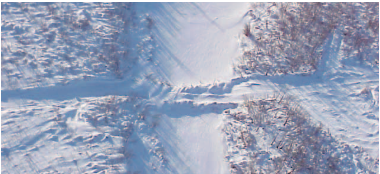
FIGURE 11. A snow fill could have been used at this stream crossing to reduce the bank height and potential for erosion under ice-free conditions.
