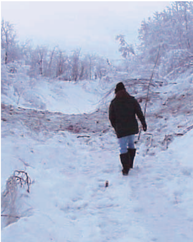
FIGURE 12. Snow fills should be constructed of clean ice or snow, creating a level surface from bank to bank. This snow fill should have been constructed with clean material and more gradual slopes.
