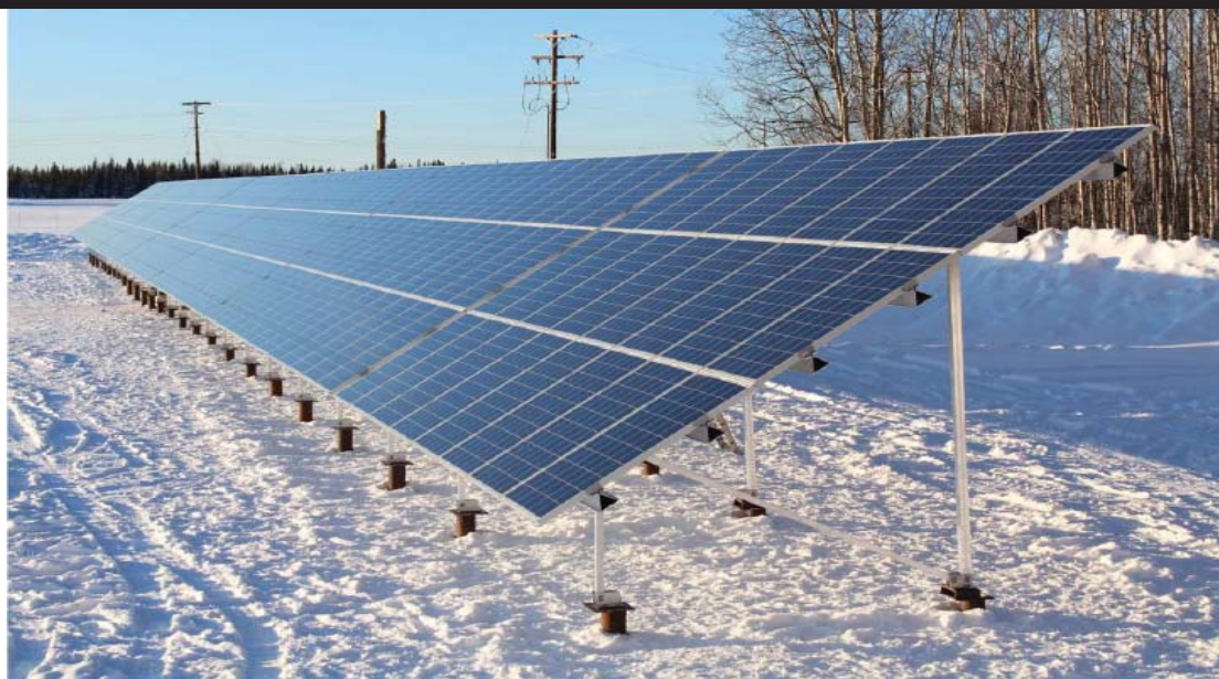
Figure 48: Solar Array at Fort Simpson - ITI
