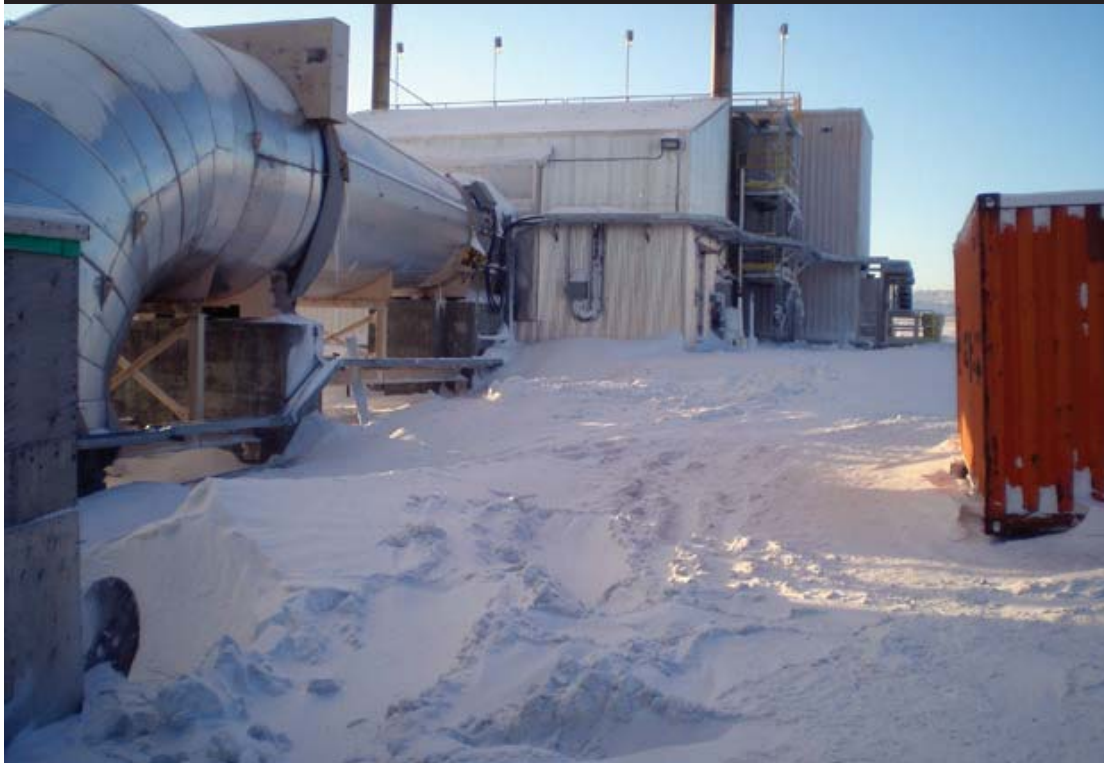
Figure 10: Underground Heat Recovery Plant at Ekati Diamond Mine - Source: International Quest Engineering Ltd.
