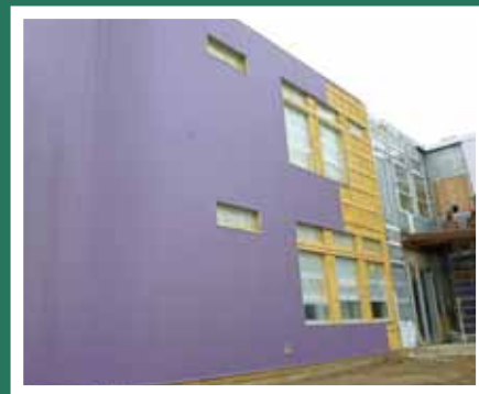
Particular attention was paid to how the new envelope was constructed at corners and fenestrations and how connections were made at parapets and footings.
