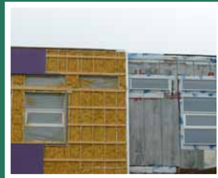
Prototype section of the building has been spray foamed and strapped, exterior cladding is being applied.
