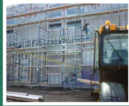
Contractors have removed the existing “skin” of the building and are beginning to apply the spray foam to the prototype section of the school.
