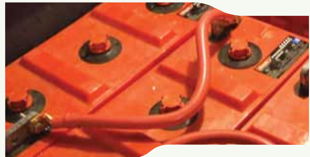
An off-grid battery bank.
