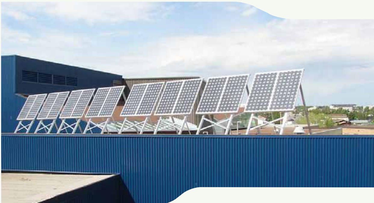
A solar panel array on top of École Sir John Franklin High School in Yellowknife.
