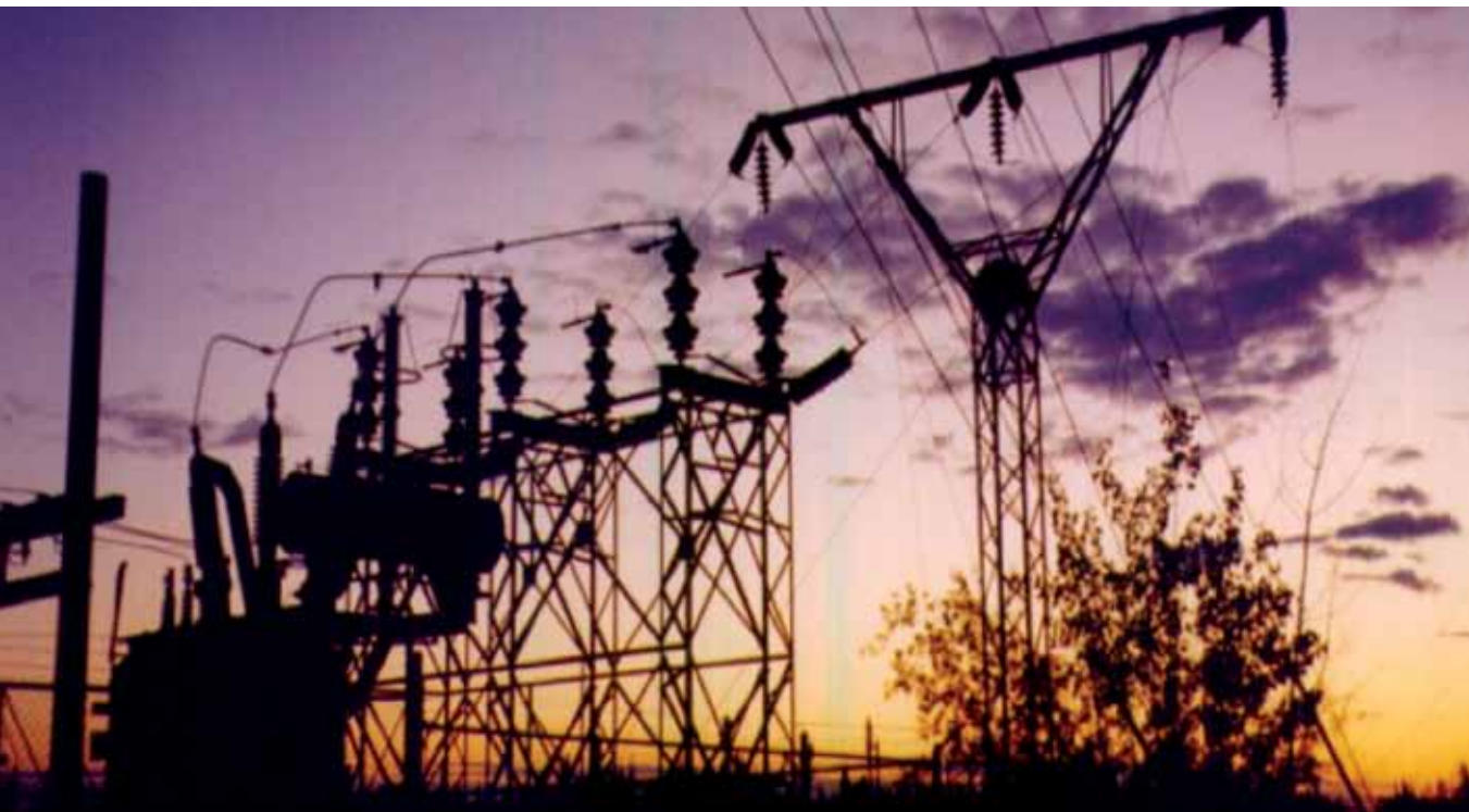
Transmission lines near Frank Channel.
