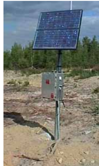
Solar panels at a Northern airport.
