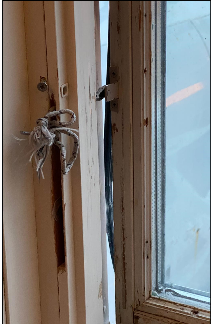
In this home, the window could no longer close. The bent window was now held with a rope, leaving a major gap that allowed in cold air, rain and snow.
