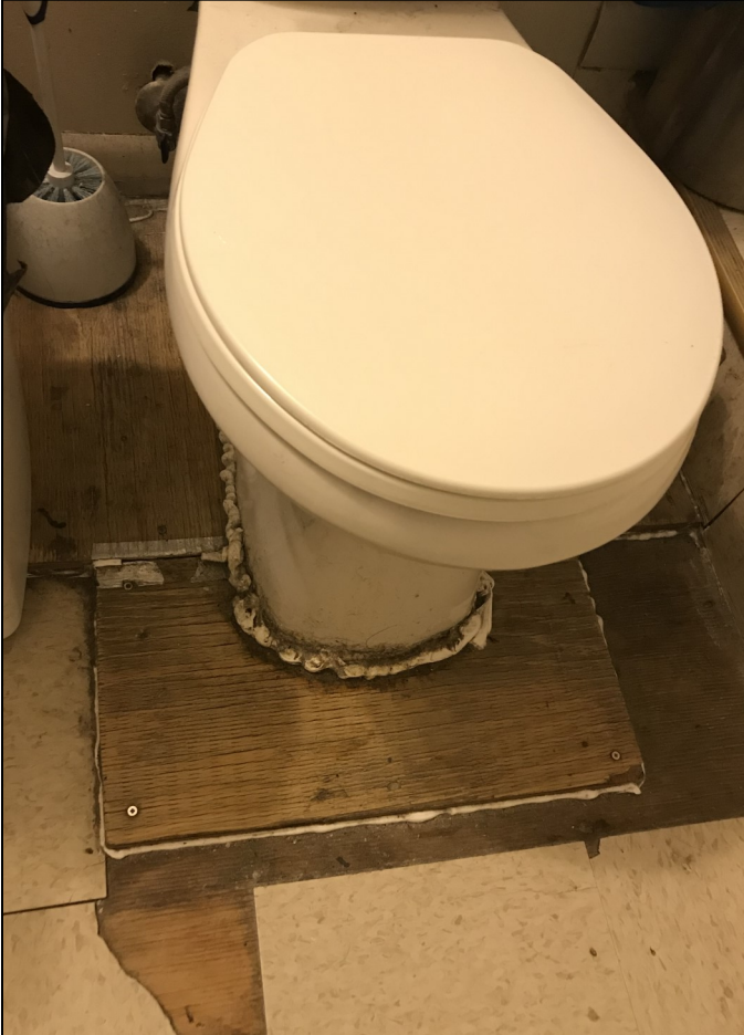
Mould, poor caulking and floors in desperate need of repair are some of the commonly needed repairs in the homes I visited.
