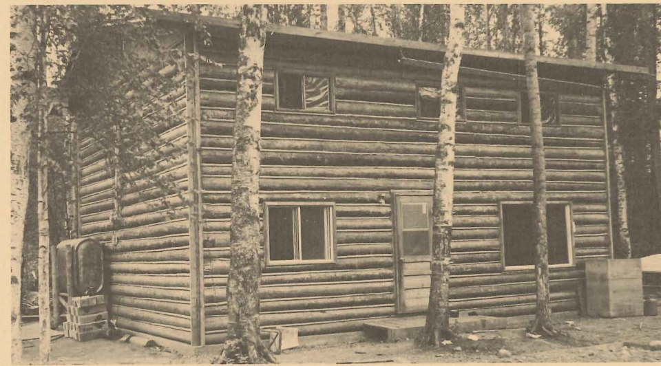
2 Don Ilich (right), secretary manager of the Rae-Edzo Housing Association, watches as Eddie Koyina installs the wiring in one of 10 public housing units built at Rae in 1976.
