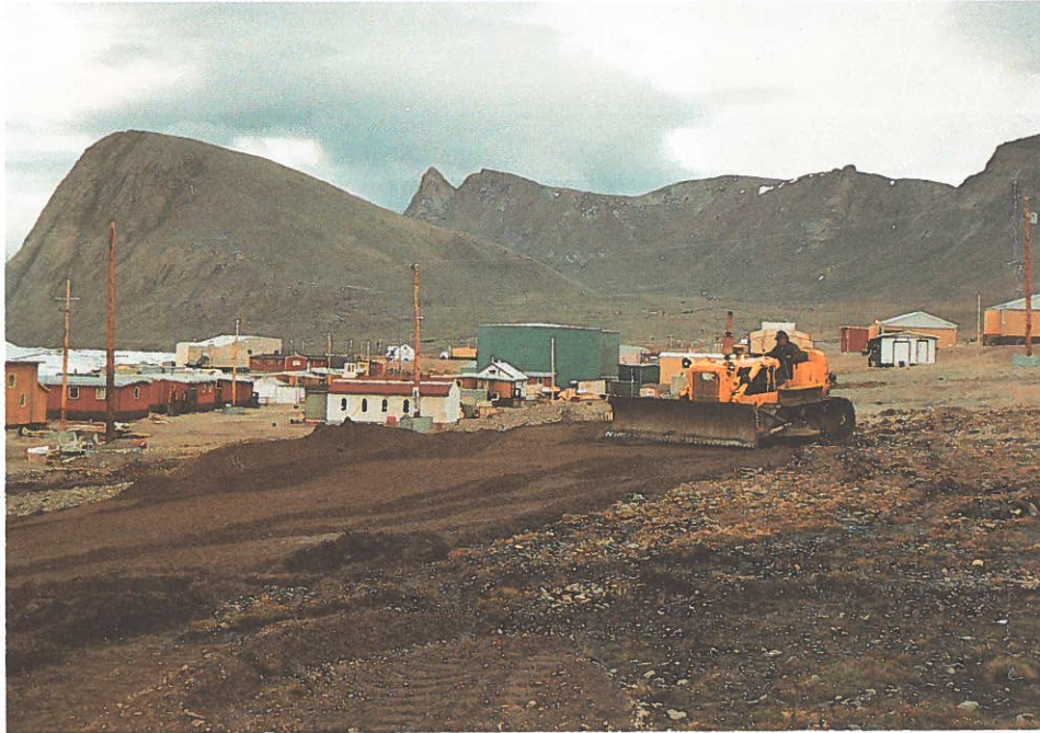
Dozer Working on First Lift (Sub-Base) of a New Road - Grise Fiord
