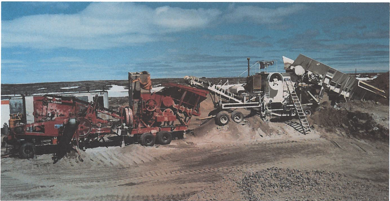
Crushing and Stockpiling Operation - Chesterfield Inlet (A Combined Water Supply/Granular Crushing Project)
