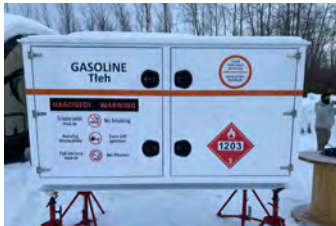
Wekweèti fuel dispenser cabinet signage in Tłıchq.
