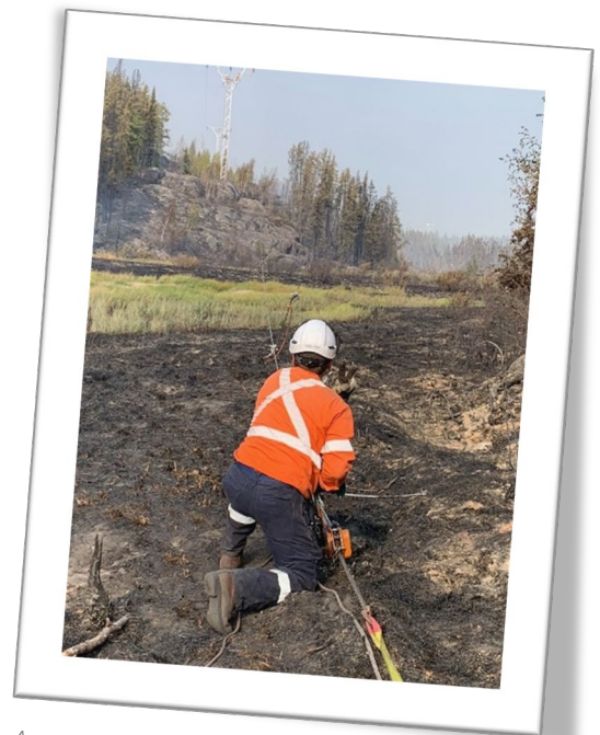
A power line technician repairs a section of the Taltson transmission line damaged by forest fires
