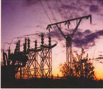
Frank Channel substation (servicing Rae/Edzo) at midnight.
