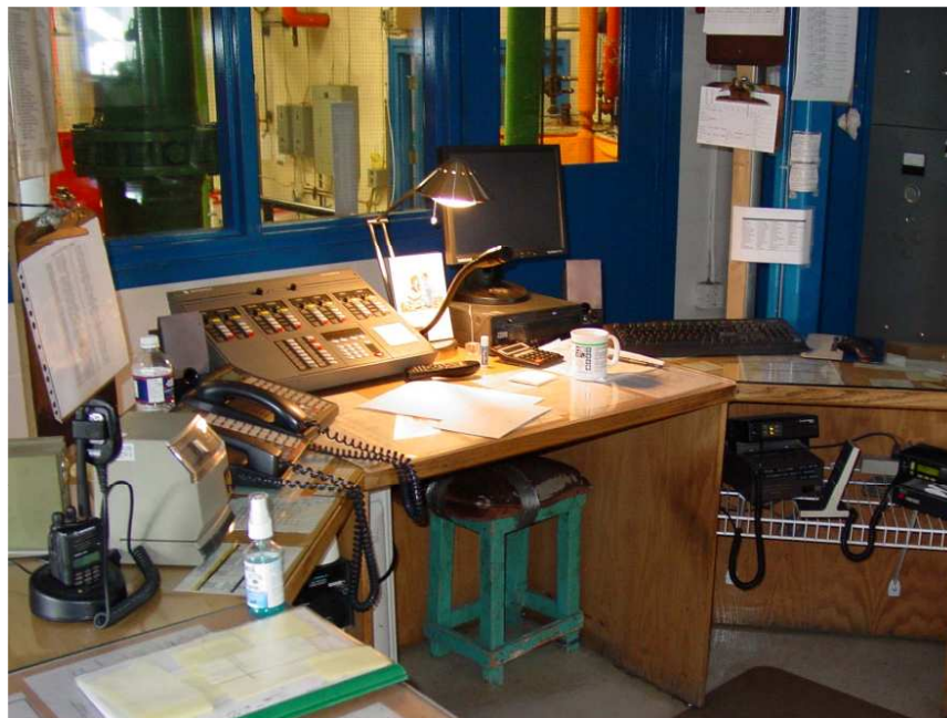
Figure A1: Fire Dispatch Equipment: Pump House
