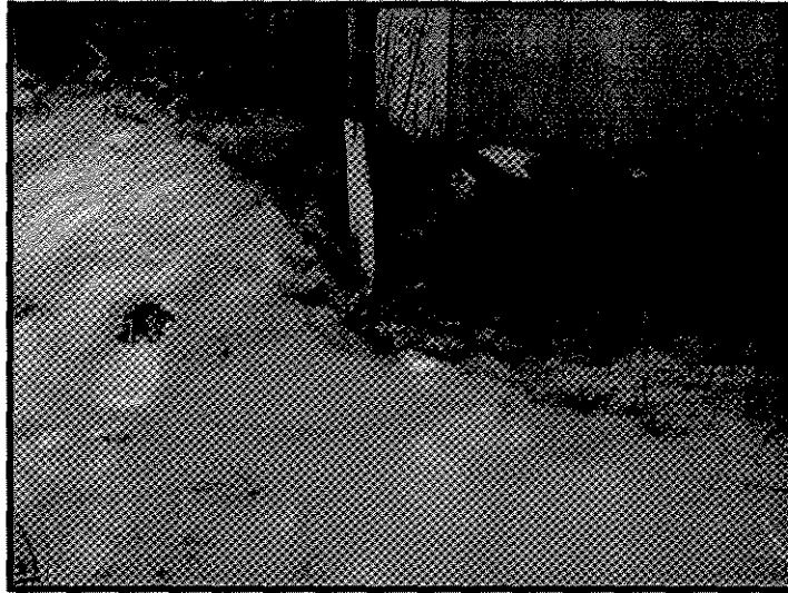
Photo 5: Depression at base of pile.
