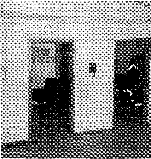
FIRE CHIEF DOOR ① COMPRESSOR ROOM ②
