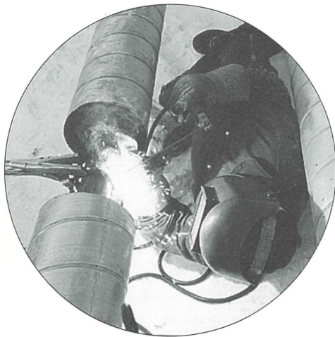
In Fort McPherson, welding continued on Aadrii Ltd.'s district heating system through the winter. The insulated pipe carries residual heat from diesel generating engines to customers in community buildings.
