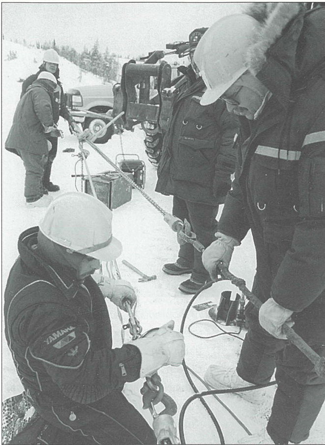
Line crews completed a critical splice repair on the Snare Yellowknife transmission line in January.
