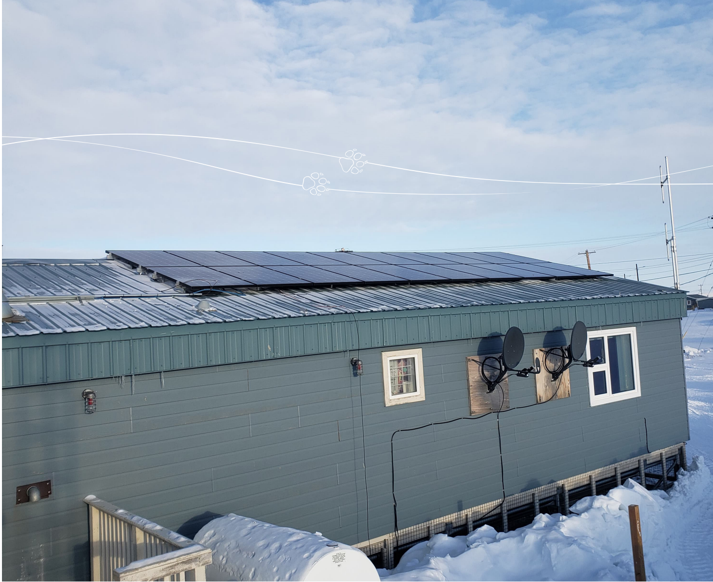
Solar panels on a building in Paulatuk
