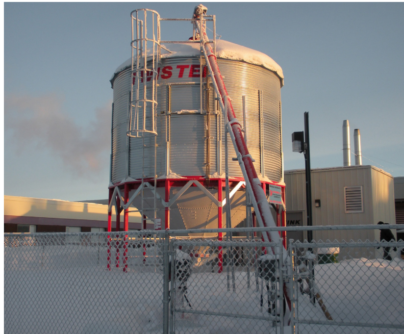
Wood pellet boiler at Chief Jimmy Bruneau School, Behchokò
