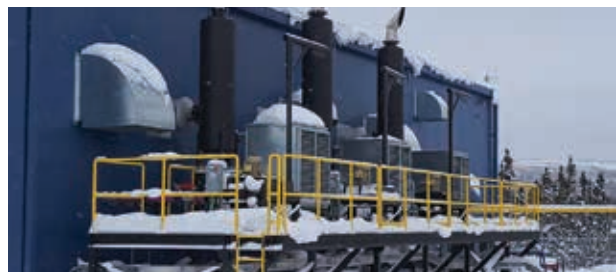
The new Łutselk'É power plant was commissioned in 2023.
