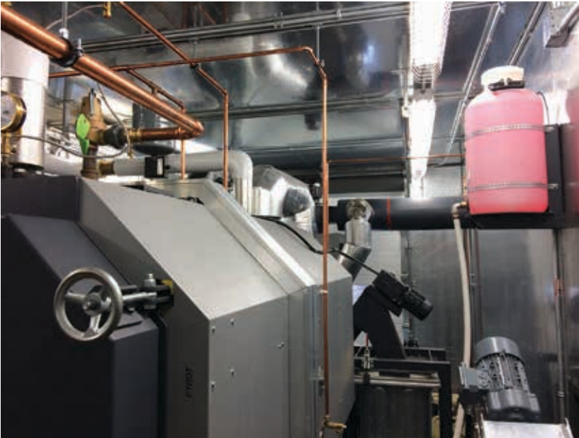
Prince of Wales Heritage Centre’s biomass heating system upgrades make it more efficient.
