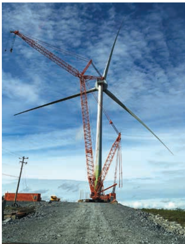
The Inuvik Wind Project is expected to reduce the town's GHG emissions by 6,000 tonnes annually.
