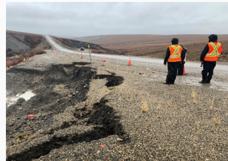
Photo: GNWT staff collaborate with other research and government organizations to monitor and study climate change impacts and adaptations for highways built on permafrost.
