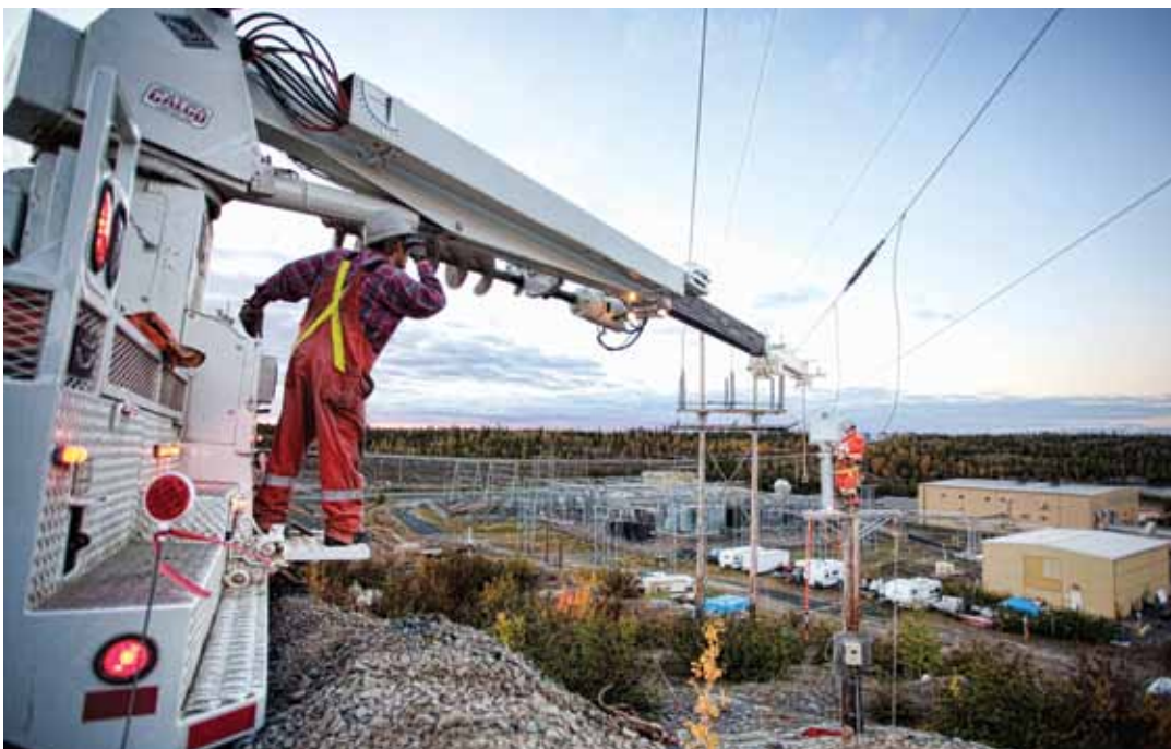
Northwest Territories Power Corporation Transmission Line
