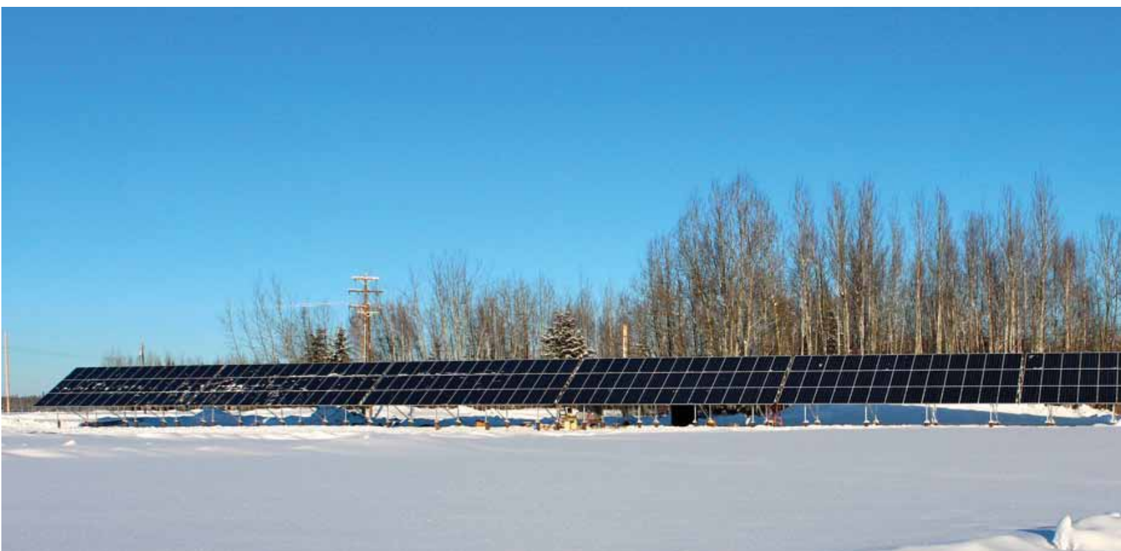
Northwest Territories Power Corporation solar installation in Fort Simpson
