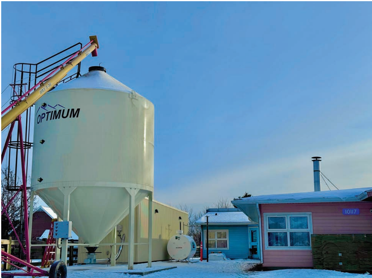
Stanley Isaiah Wood Pellet Silo and Boiler Container
