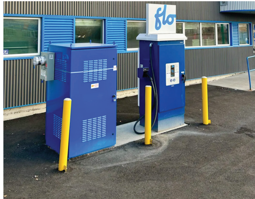
EV Fast Chargers Installed by Naka Power in Yellowknife
